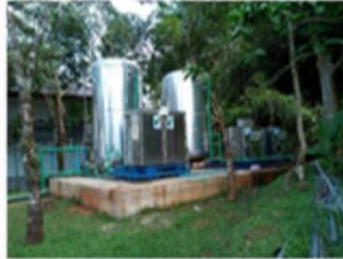
Hot water from Heat pump
