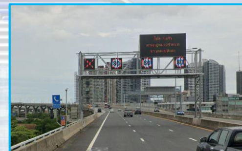
VMS Traffic Sign Board
